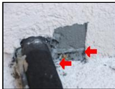
3.4 Picture 2 A/C Freon Lines
