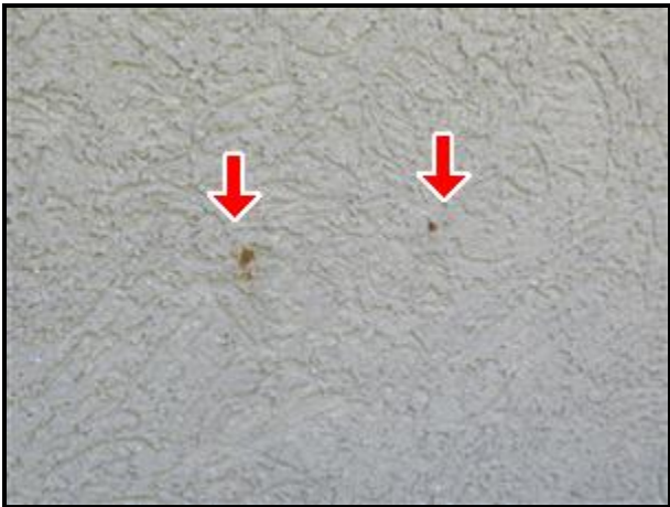
9.4 Picture 5 Rust Spots
