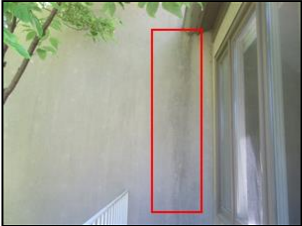
9.4 Picture 3 Under Missing Rear Kickout
