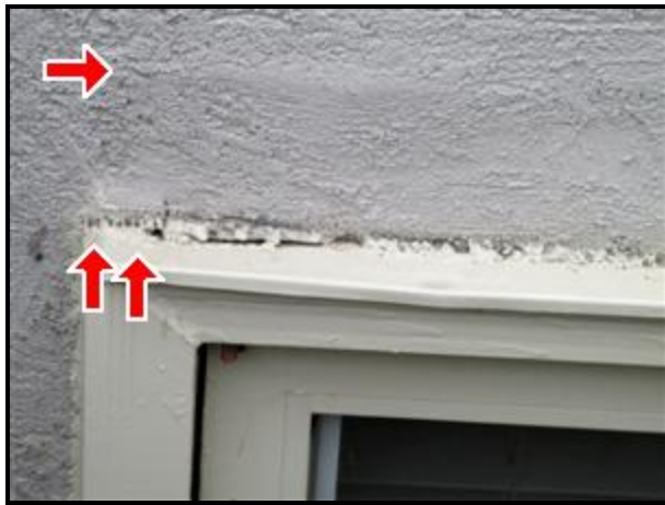
2.2 Picture 1 Exposed Mesh & Bulge
