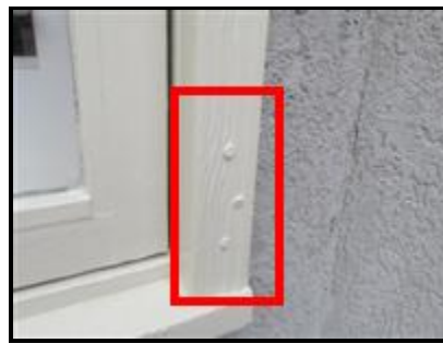
5.0 Picture 2 Previous Repair - Left Side
