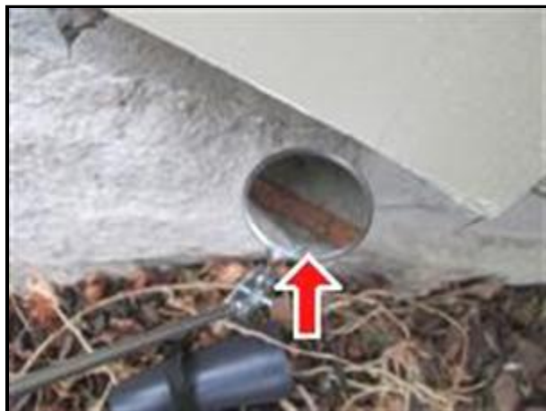
2.4 Picture 1 Foam Under Wall
