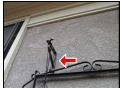
9.0 Picture 6 Rear / Screws in Stucco
