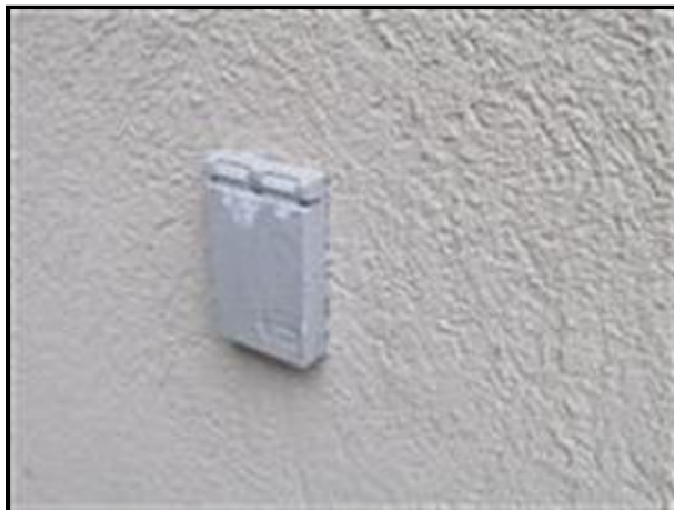
3.2 Picture 1 Example of Breach
