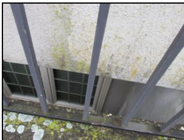
9.1 Picture 4 Mold by Daylight Window
